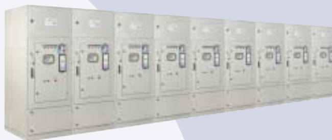
Medium Voltage MCC formation with Load Make Fault Break switches
